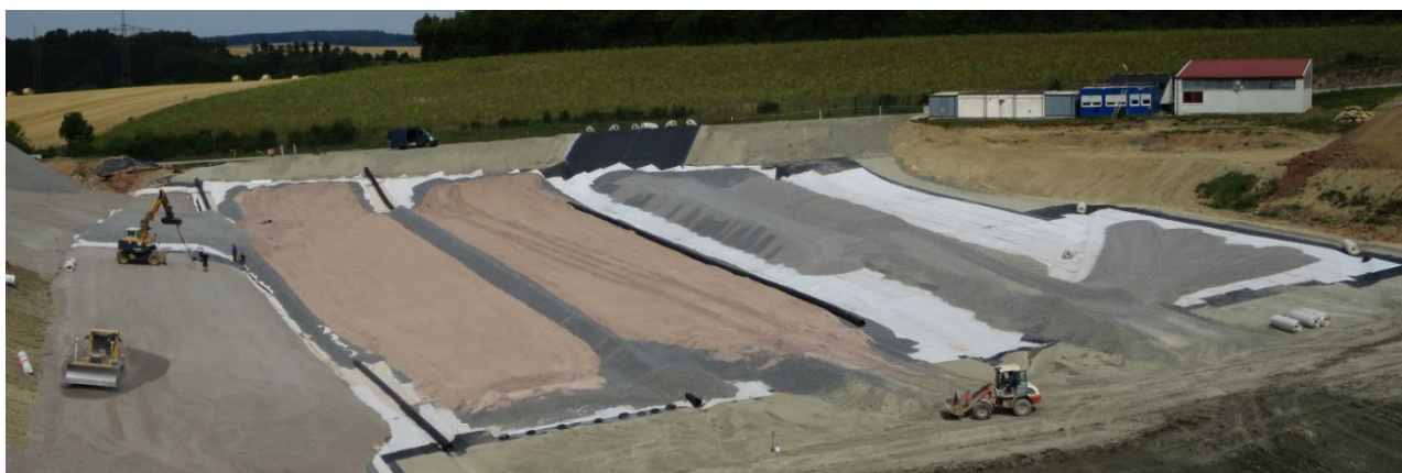
Figure 12: Preparation of a landfill site for the subsequent dumping of conventional and cleared waste (waste management company of the district of Neckar-Odenwald (AWN – Abfallwirtschaftsgesellschaft des Neckar-Odenwald-Kreises mbH)
